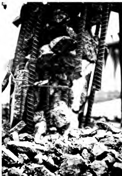
Photo 26. Some vertical reinforcing steel in tied columns broke, usually near the weld splicing bars as shown here.
